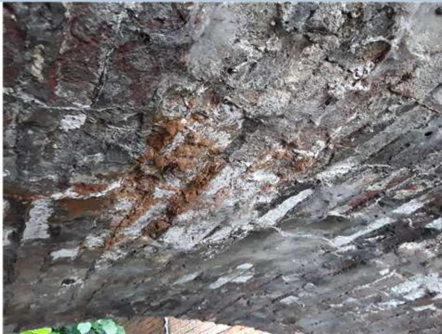
Crown - Example of Historic Seepage Seepage through brickwork evident in leachate and calcite deposits on brick faces.
