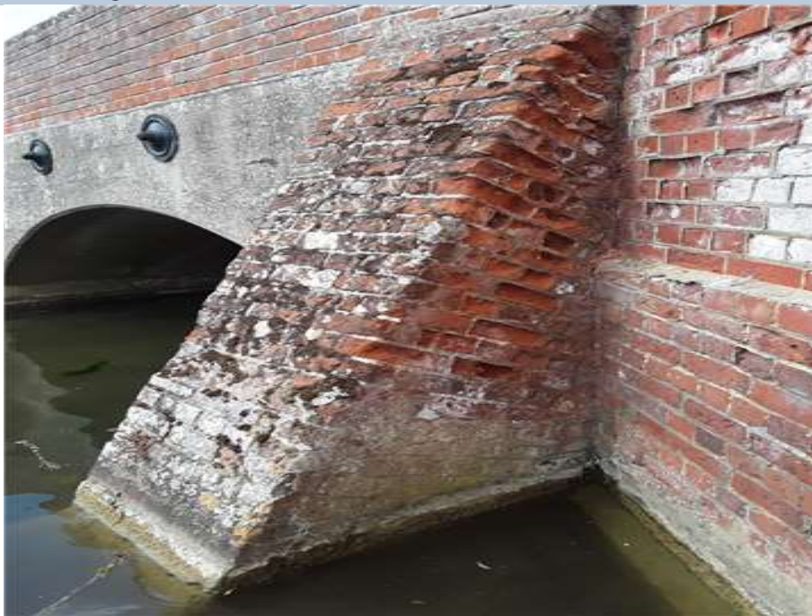
South East Buttness - Moderately Weathered Brickwork Both Buttnesses have moderate weathering to brick work.
