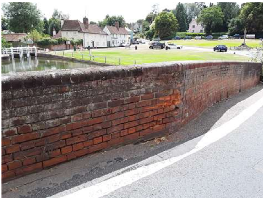
South Parapet Moderate loss of pointing to lower courses of inside face.
