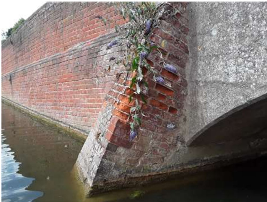
South West Buttness - Vegetation Weeds/ Shrub growing from South West abutment. Plant is Buddleia (Butterfly Bush) and will likely contribute to deterioration of brickwork.
